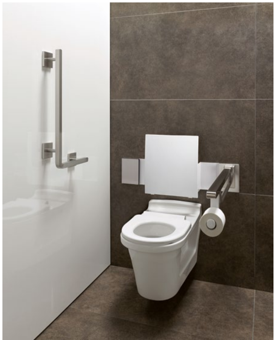
WC CF wandhängend, barrierefrei (CW142Y) WC CF wall-hung, barrier-free (CW142Y)
